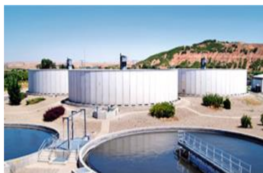
1. First stage biological filters
